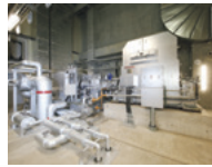
5 Steam turbine generator
