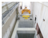
8 Ash pit and ash crane operation room
